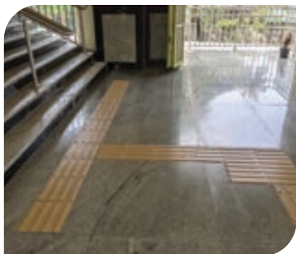
Improperly laid tactile tiles (Indoor)
