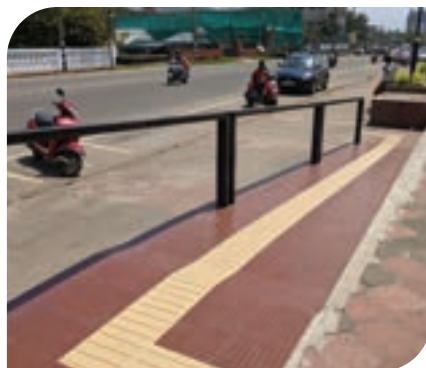
Improperly laid tactile tiles (Outdoor)
