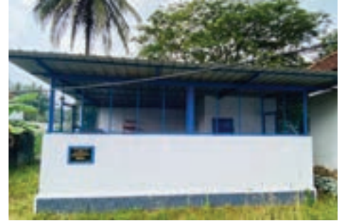
The flood damaged the MT SHS at Neerattupuram. ESAF constructed a kitchen and mess hall with the support of ESAF SFB.
